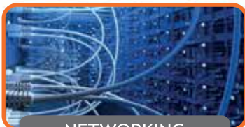
NETWORKING CCTV / DATA
